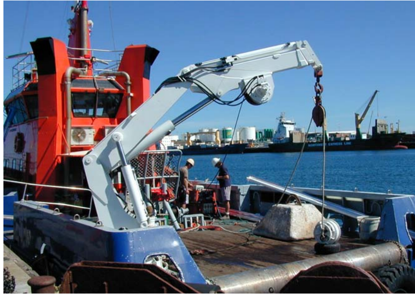
Figure 3: Back deck of FP Response. Note the hydraulic crane in the foreground, concrete mooring block and in the background, the hydraulic winch and generator.
